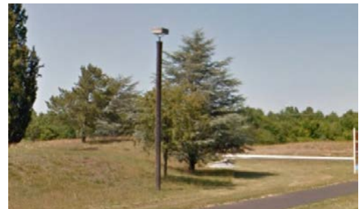
Figure 59 Existing trail lighting at Park Road intersection with partial cut-off fixture that hides the light source and a pole with duplex finish (color applied)
