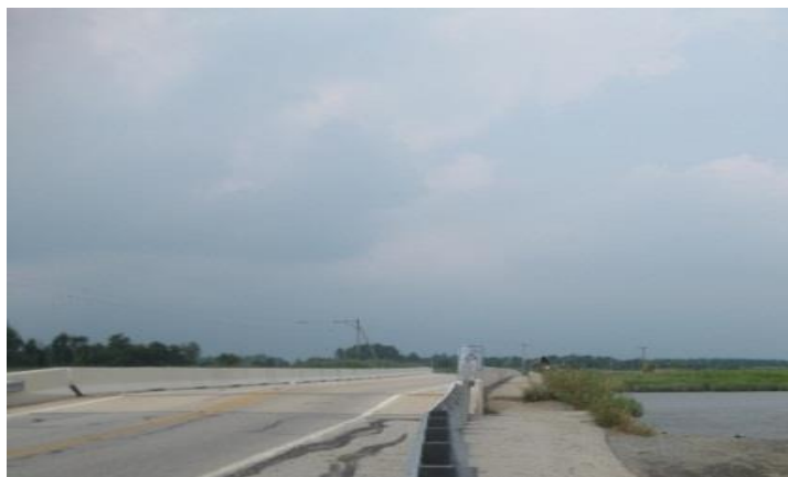
Some of the Bridges on State Route 9 have provisions for fishing built in to them.
